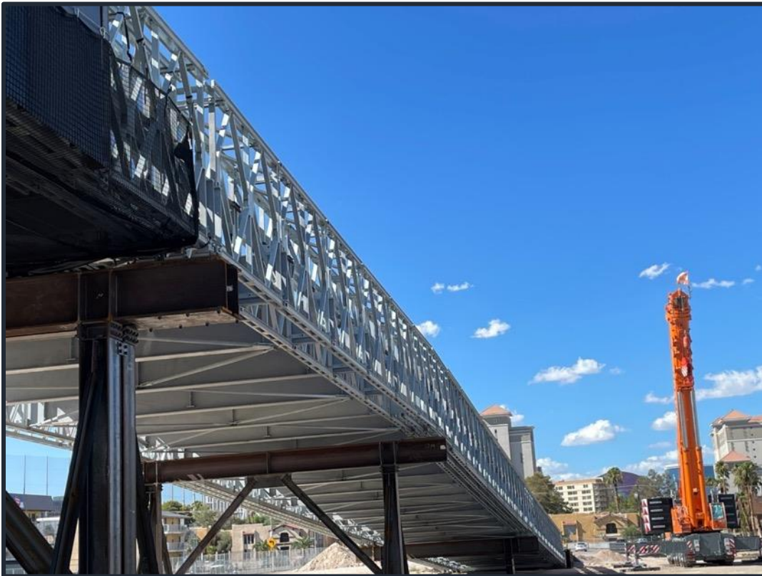
One of two primary vehicle bridges designed off site for the event.
